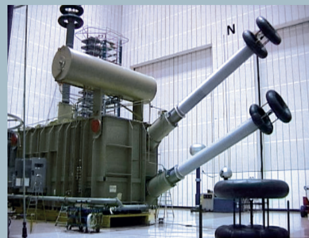
Fig. 7: 283,7 MVA/Yy single phase transformer for China with two valve bushings arranged at the front side of a tank.
