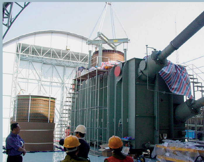
Fig. 13: "Old" winding block being taken out of the dismantled transformer with the help of a truck crane (the new winding block is waiting on the left hand side).
