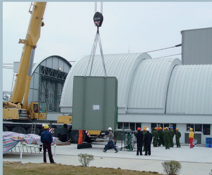
Fig. 12: Repair hall at TSQ Station (with the roof re-moving, so the tank containing the new winding block can be lifted into the hall).
